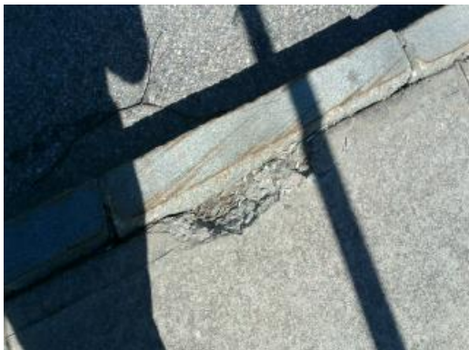
Site - Damaged Concrete Walks
