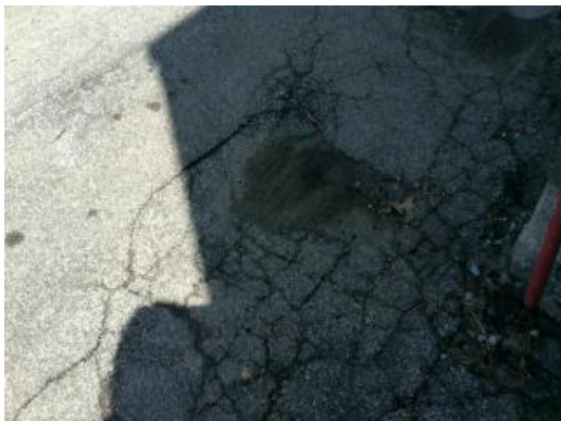
Cracked Asphalt Paving
