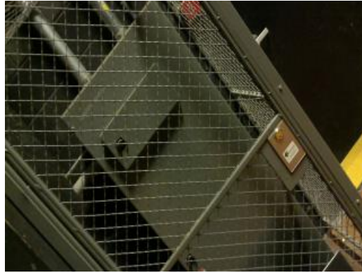
Main Building - Transfer Switch
