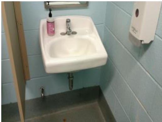
Main Building - Aged Restroom Sink
