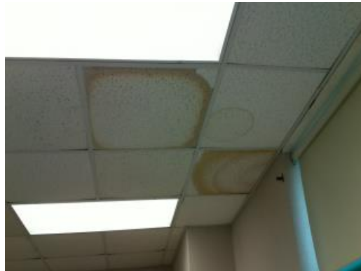
Stained Ceiling Tiles
