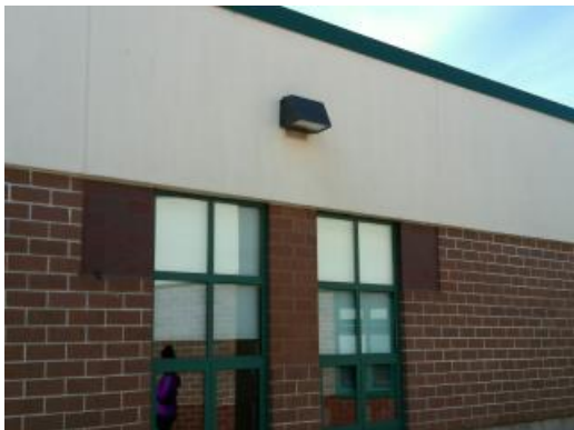
Building Mounted Light
