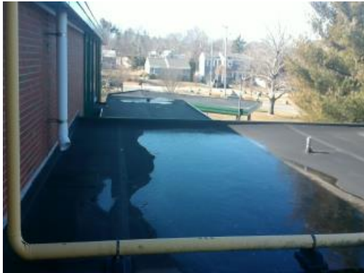
Ponding On Roof
