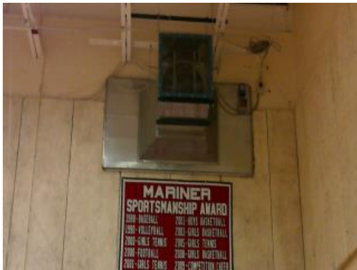
Main Building - Aged Gym Make-up Air Unit
