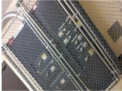
Main Building - 1200 Amp Switchgear
