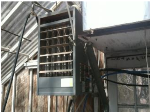
Building 03 - Aged Unit Heater
