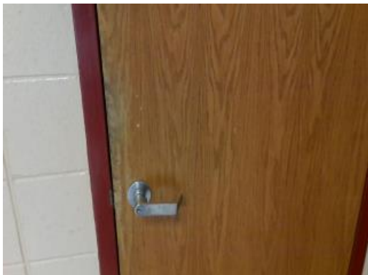
Damaged Interior Wood Door
