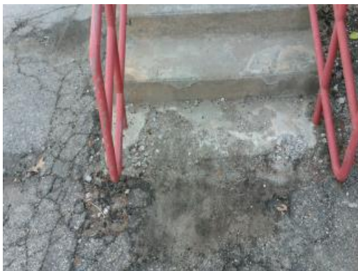
Damaged Concrete Stairs
