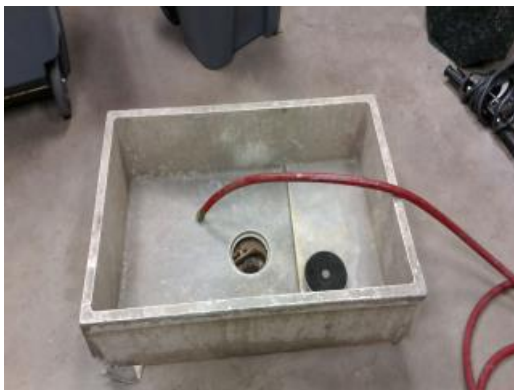
Main Building - Stained Mop Sink
