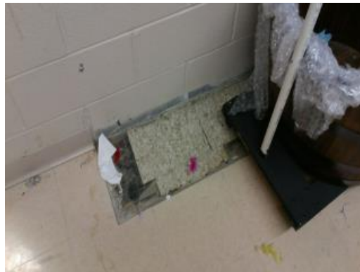
Main Building - Missing And Broken VCT Flooring
