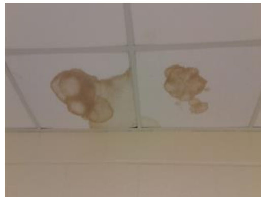
Main Building - Stained Ceiling Tiles
