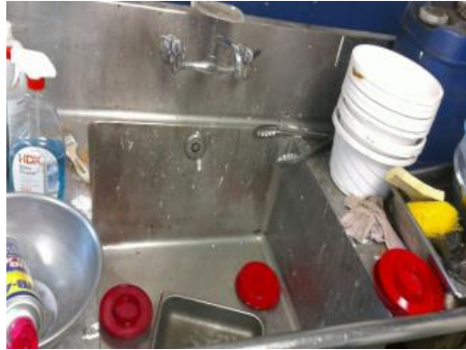
Building 03 - Stained Utility Sink
