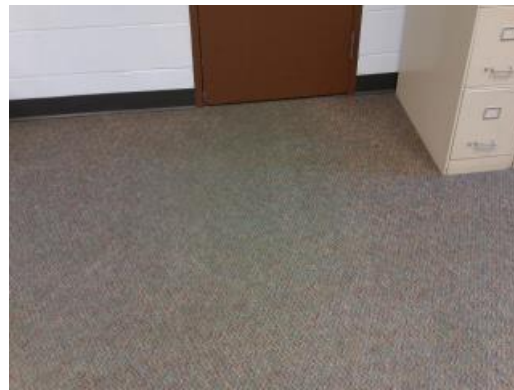
Main Building - Worn Carpet
