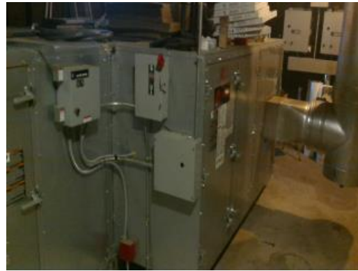
Main Building - Aged Indoor AHU
