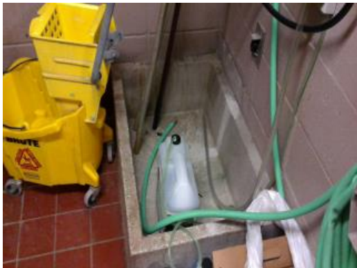
Corroded Mop Sink
