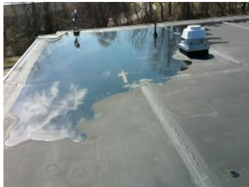
Main Building - Ponding On Roof
