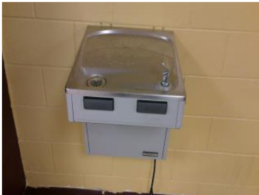
Main Building - Refrigerated Water Fountain
