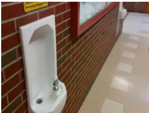
Inoperable Drinking Fountain
