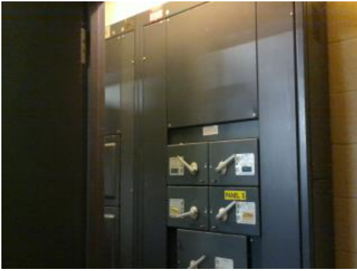
Main Building - 2000 Amp Switchgear
