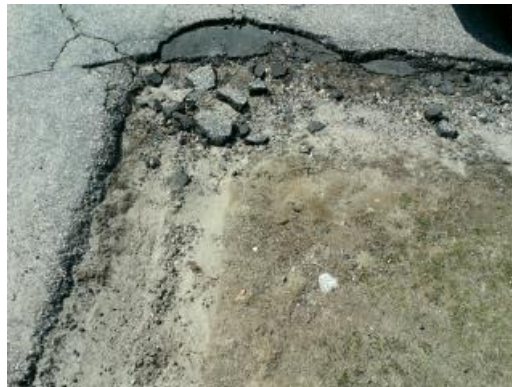
Deteriorated Asphalt Paving
