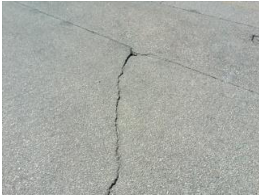
Site - Cracked Parking Lot Paving
