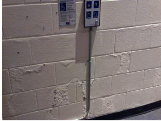
Damaged Paint On CMU Wall
