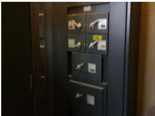
Main Building - 3000 Amp Switchgear
