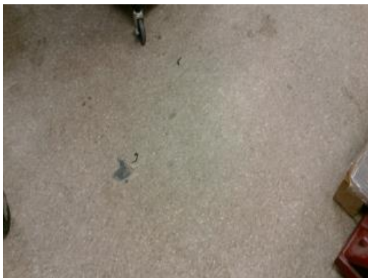
Main Building - Worn VCT Flooring
