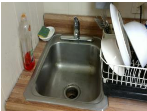
Main Building - Aged Classroom Sink
