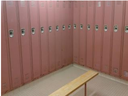
Worn Paint On Lockers
