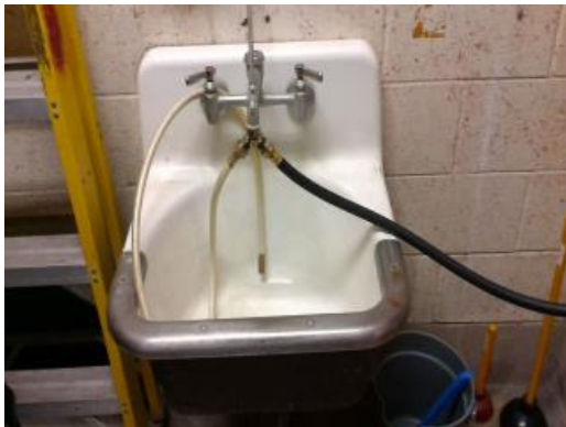
Main Building - Typical Service Sink
