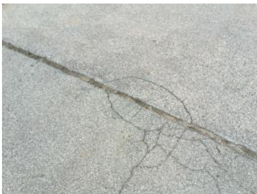
Cracking Sidewalk Paving
