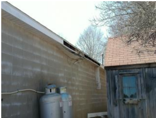
Building 03 - Damaged Soffit
