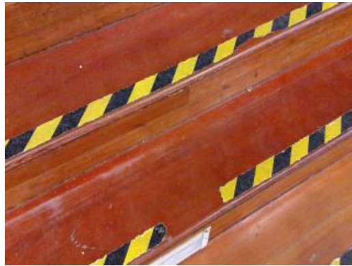
Missing Stair Tread
