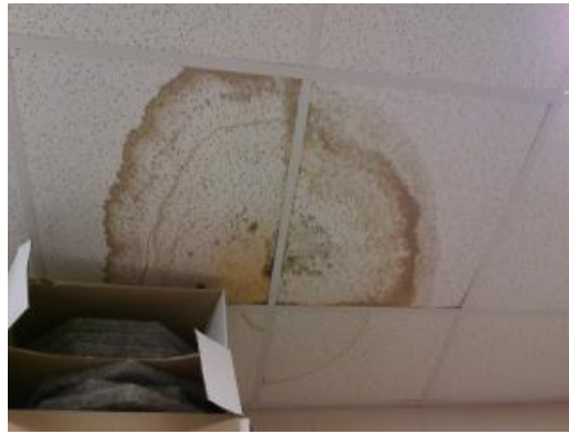
Main Building - Stained Ceiling Tiles
