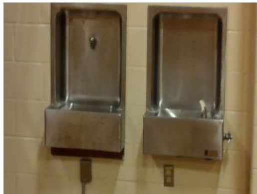
Stained And Aged Water Fountains
