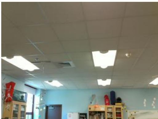
Main Building - Lighting Fixtures
