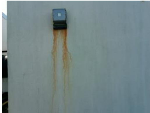
Main Building - Stained Stucco
