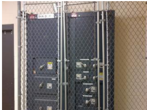
Main Building - 800 Amp Switchgear
