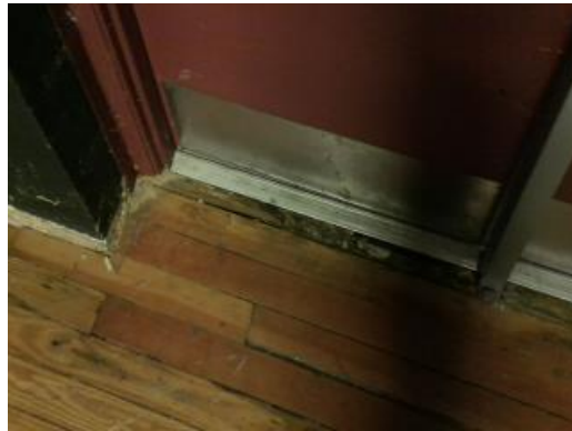
Main Building - Worn And Splitting Wood Plank Flooring
