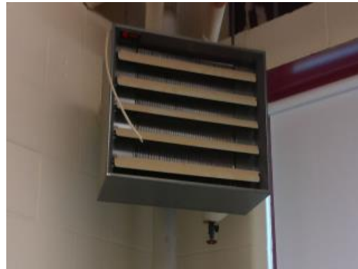
Main Building - Original Unit Heater
