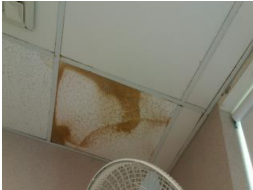
Stained Ceiling Tile
