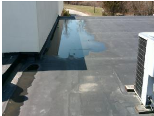
Ponding On Roof
